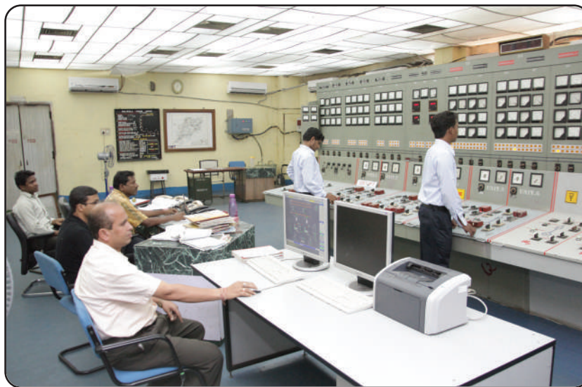
Main Control Room of BHEP, Balimela
